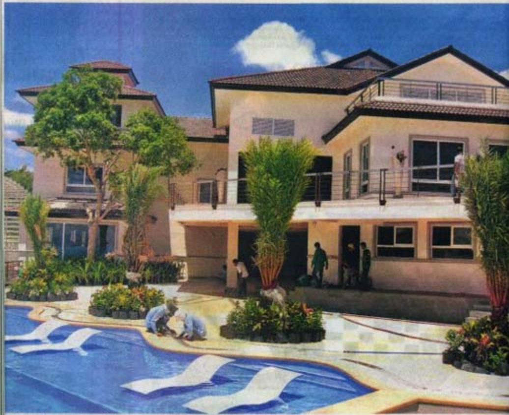
STILL WATERS: Workers giving the finishing touches to a high-end villa complete with a swimming pool and garden
